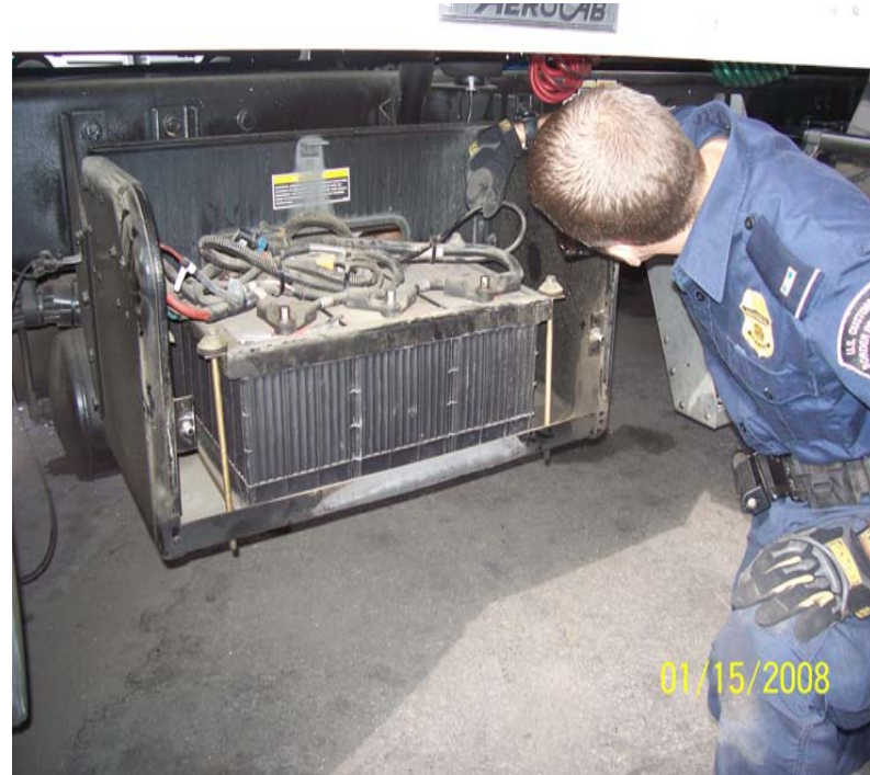
Battery Area / Secure
