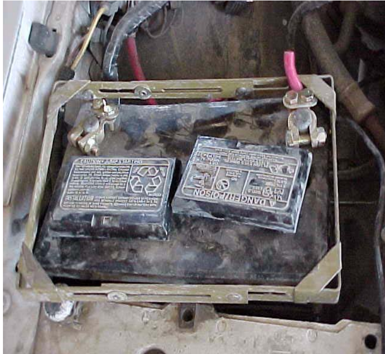
Top Cover Loose / Not Wired
