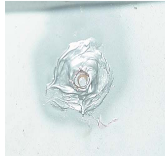
Putty Inside Door / Unusual
