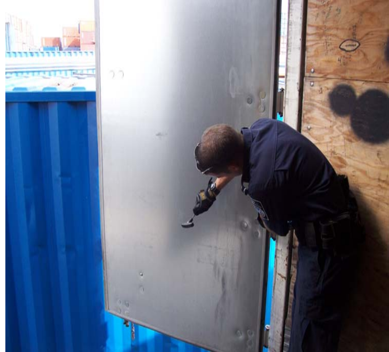
Repairs / Weld Marks
